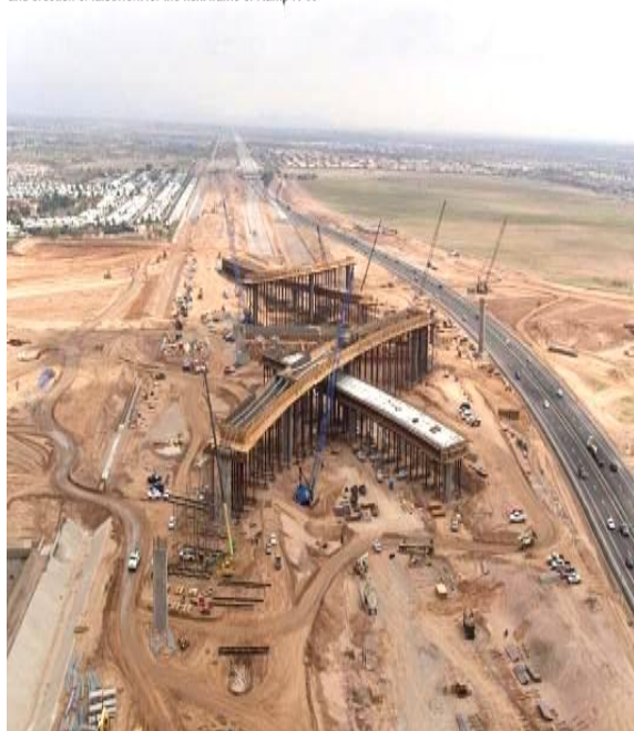
3/2/04 - Looking E along US 60 at the bridge construction and erection of falsework for the next frame of Ramp N-W
